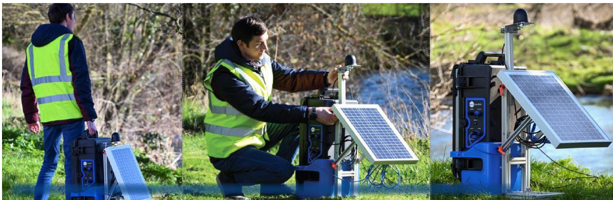
Aquamonitrix® mobile unit powered by a solar/battery pack
